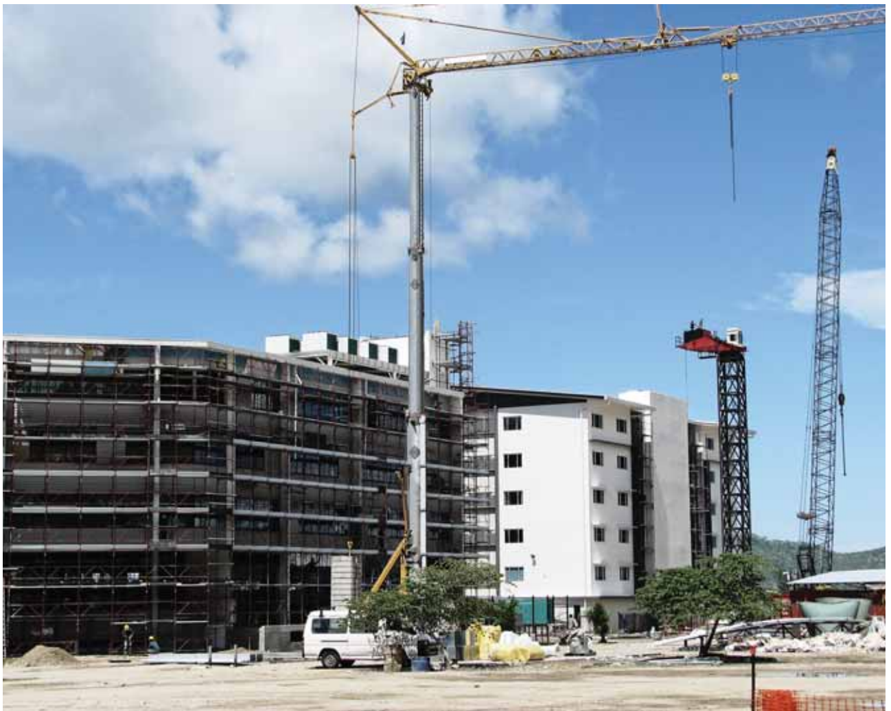
NEW APARTMENTS AND OFFICE BUILDINGS UNDER CONSTRUCTION AT HARBOUR CITY, JUST OUTSIDE PORT MORESBY'S CBD.
